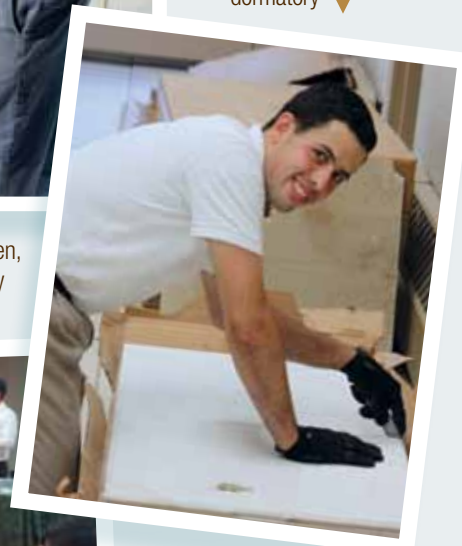
Br. Grant Tavarez works to lower the ceilings to conserve heat in the dormitory ▼
